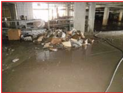
▲ The debris and mud left behind
